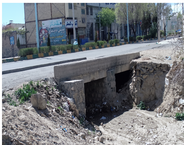
Fig. (14). Bridge openings are blocked.
