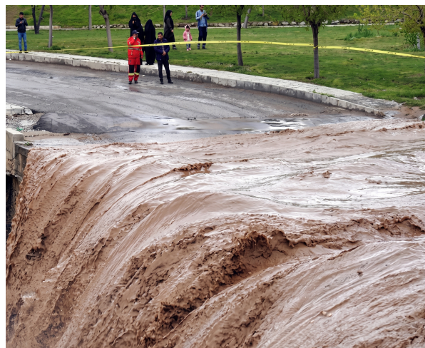
Fig. (15). Creating a narrow path for the waterway due to the construction of a bridge and its narrow span.
