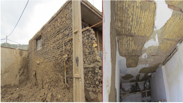
Fig. (6). The building with a load-bearing wall system supported by a steel coil and a rough brick arch roof; the adjacent building, which lacked a suitable structural system, was destroyed.
