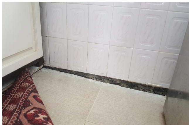
Fig. (13). Excessive settlement of the kitchen floor due to the use of soil instead of rubble (blockage).
