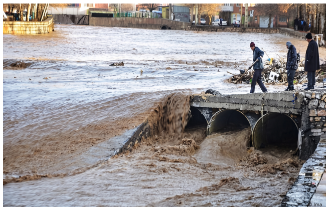
Fig. (12). A narrow path being created for the waterway due to the construction of a bridge and its narrow span.
