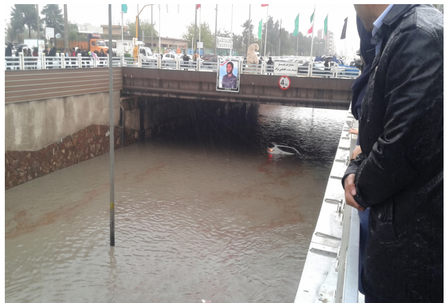
Fig. (11). Construction of an underpass without considering the drainage system of the water entering the underpass, the steep slope of the underpass, and the accumulation of inlet water.
