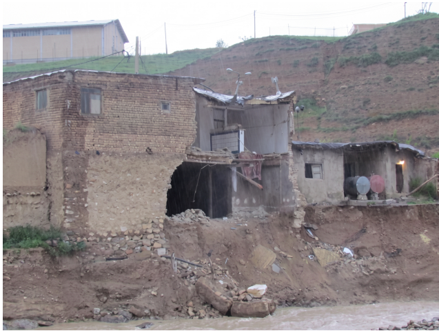
Fig. (7). Foundation scouring and collapse of the load-bearing walls and roof.
