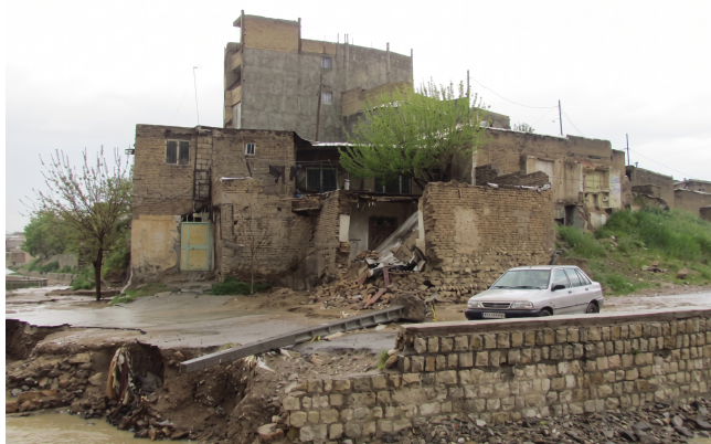
Fig. (4). Residential buildings lacking design considerations for flood load and proper technical specifications are more vulnerable along the flood route.
