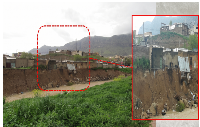
Fig. (5). Residential construction along the river upstream route, which has scoured the foundation and destroyed the buildings during the flood.
